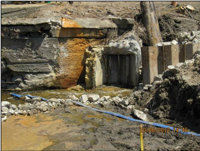
June 20, 2012: Water exiting bypass pipe
